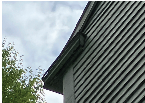
Image A-22: Detail of deteriorated wood cornice
