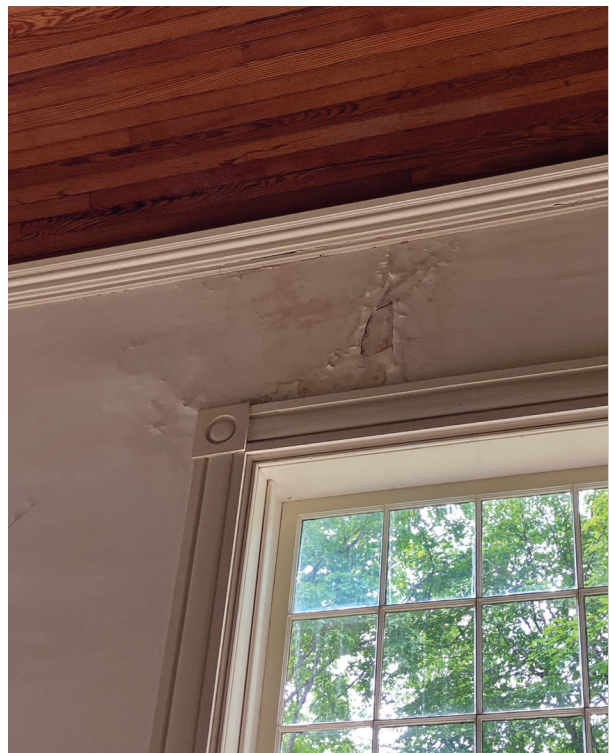
Image B-07: Interior plaster disruption betraying water damage and roof leakage
