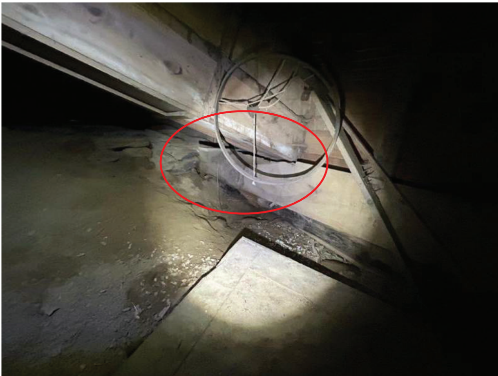
Photo 14 Partially rotted beam in soil below wall
