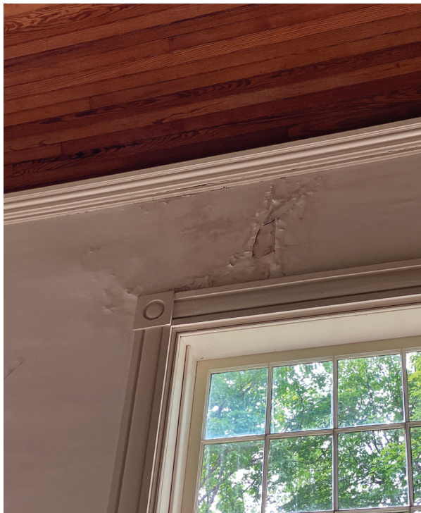
Image A-07: Detail of interior plaster and paint damage indicates leak location
