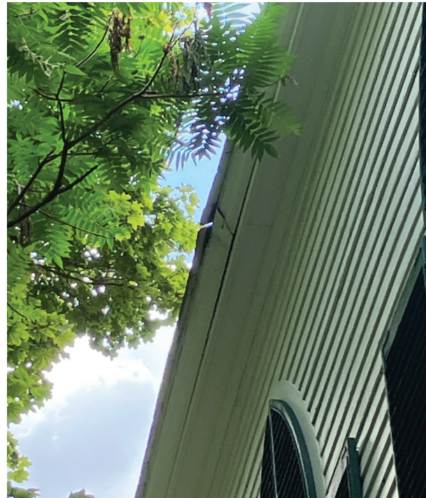
Image A-08: Suspected leak location at deteriorated cornice
