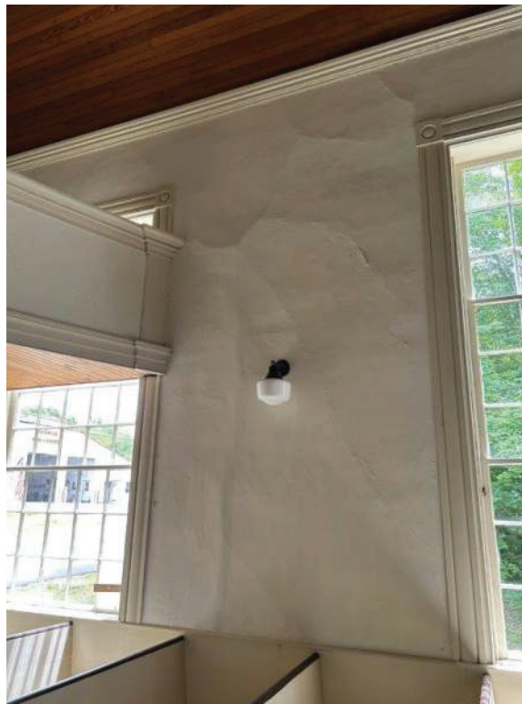
Photo 20 Diagonal shear cracks at end of balcony
