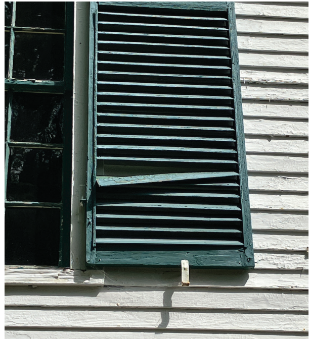
Image A-25: Existing shutters are mostly in goof condition, with some loose blades
