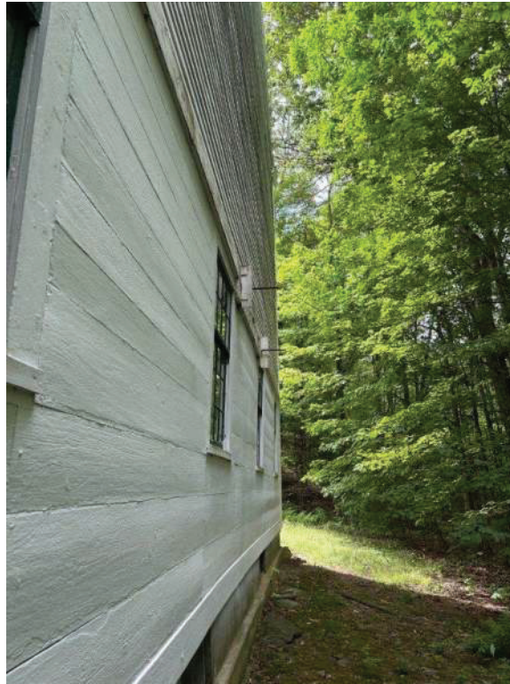
Photo 7 Outward bowing west elevation with past wall reinforcement rods
