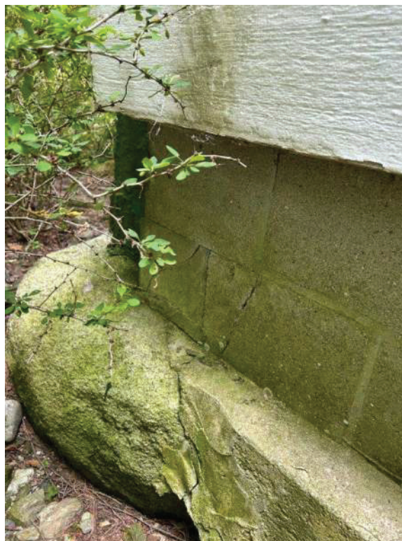
Photo 8 Step cracks at northwest corner of foundation
