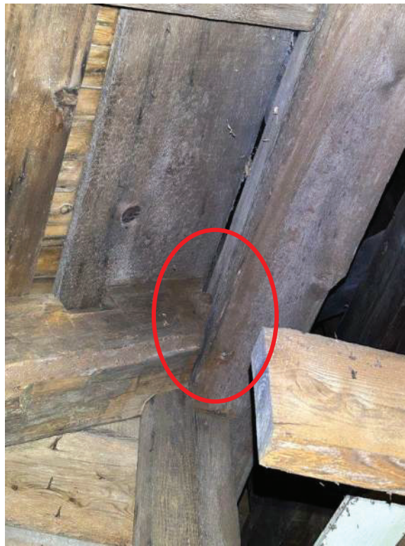
Photo 24 Roof rafter pulling out from mortise
