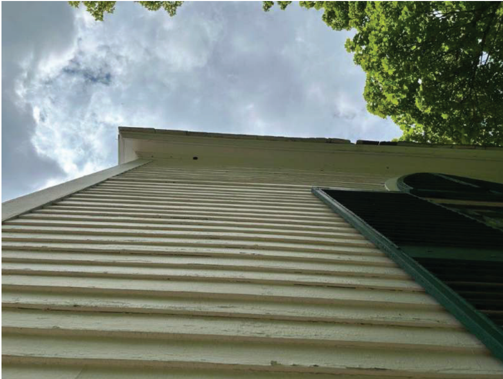
Photo 11 Hole in soffit board
