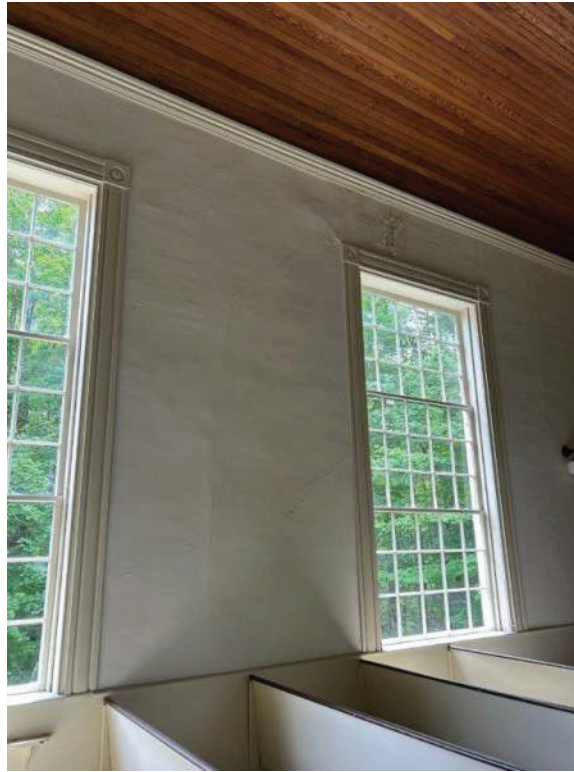
Photo 19 Past water damage over window
