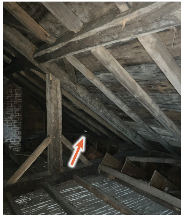
Image A-09: Daylight is observed in attic interior, indicated with arrow.
