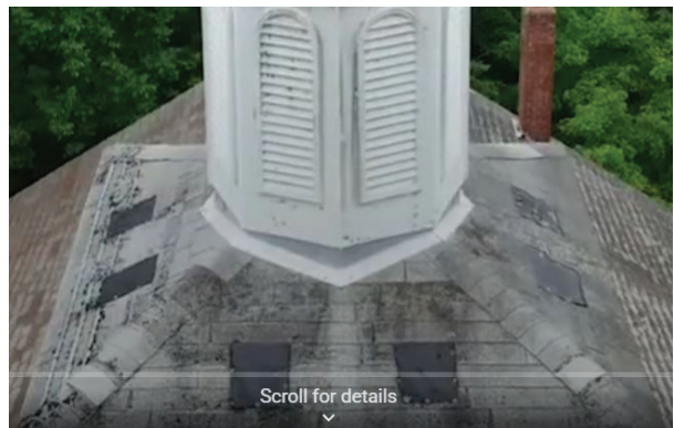
Image A-05: Drone shows poor condition of the belfry roof
