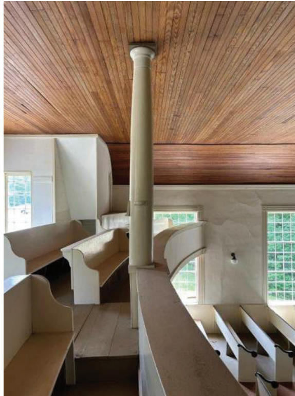
Photo 21 Tilted column support at balcony
