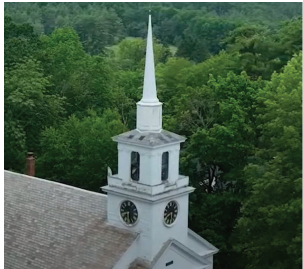
Image A-04: Owner-provided drone footage showing steeple condition
