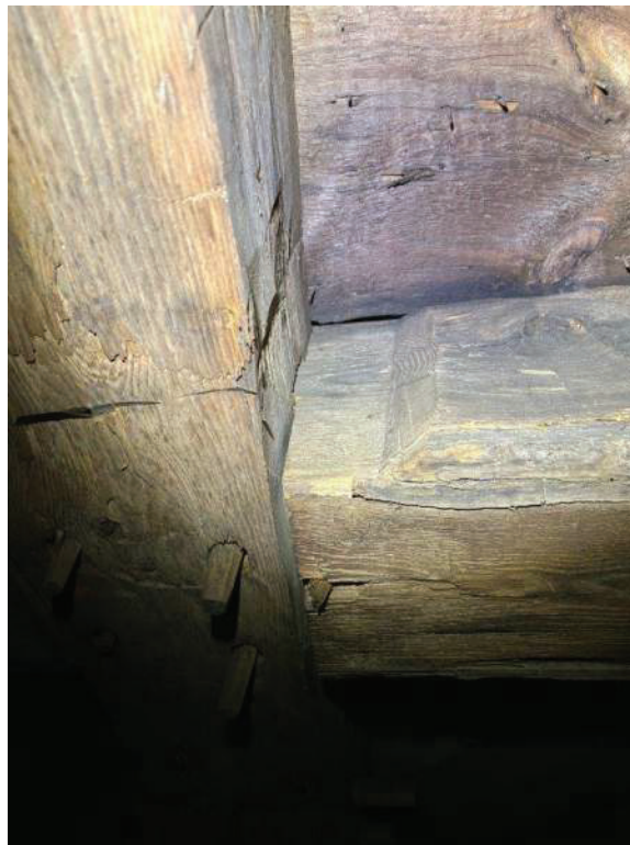
Photo 22 Typical notch at roof purlin
