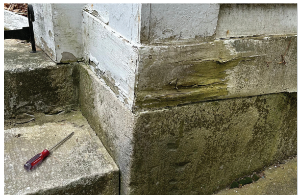
Image A-21: Deterioration of wood watertable trim in contact with masonry
