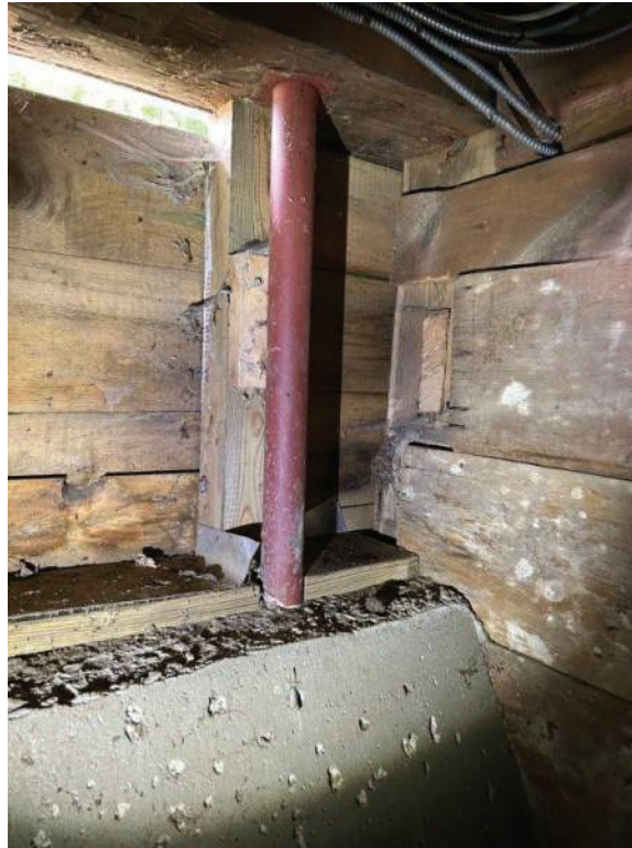
Photo 15 Lally column with poor cap plate and rusting base
