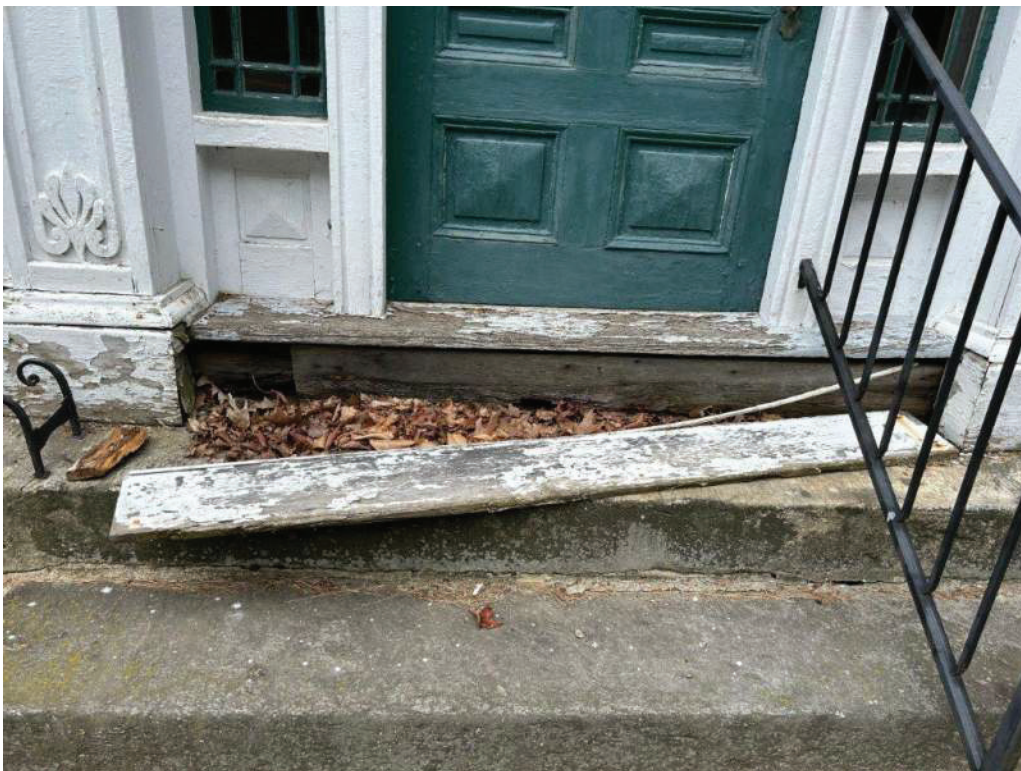
Photo 2 Eroded mortar joints, damaged trim, and rotted sill plate
