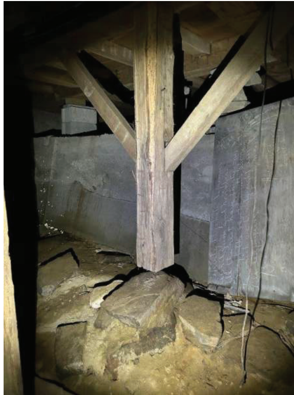
Photo 13 Unsupported post end
