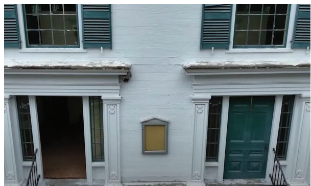
Image A-06: Drone photo shows the poor condition of the flashing of the door entablatures
