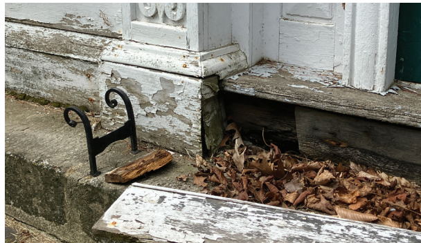
Image A-20: Wood trim in contact with masonry is deteriorated
