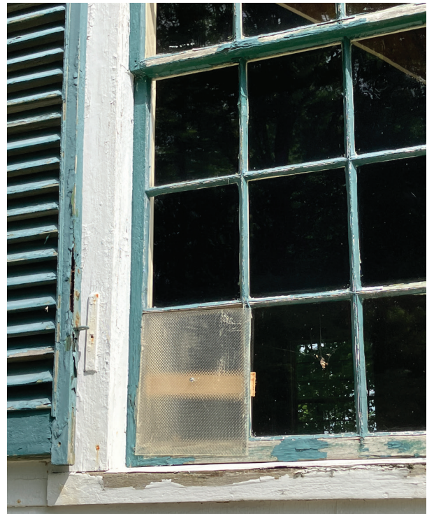
Image A-29: Existing windows have glazing putty failure but are generally structurally sound
