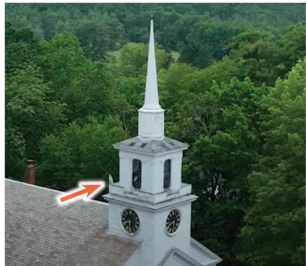
Image A-11: Only one of the original acroteria remains, indicated with arrow
