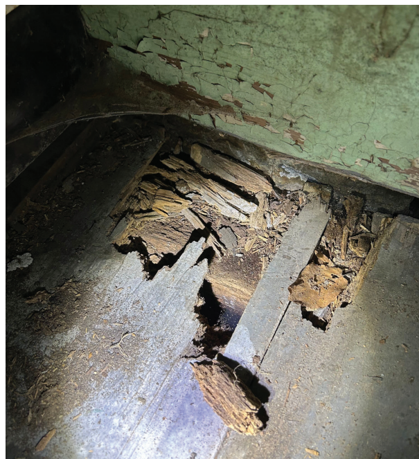
Image B-11: Deteriorated floor
