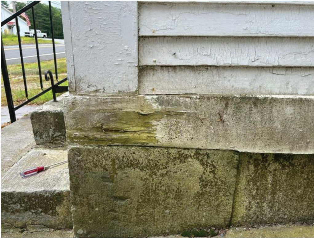
Photo 3 Crushing and rotted sill plate
