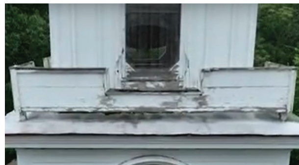
Image A-12: Drone footage gives a detailed view of deteriorated existing wood balustrade at the clock pavilion roof
