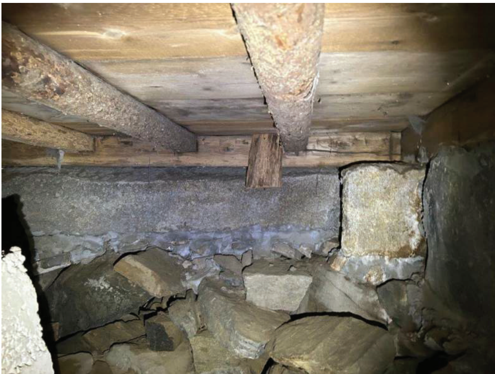
Photo 12 Uneven bearing surface for sill plate contributing to rotation
