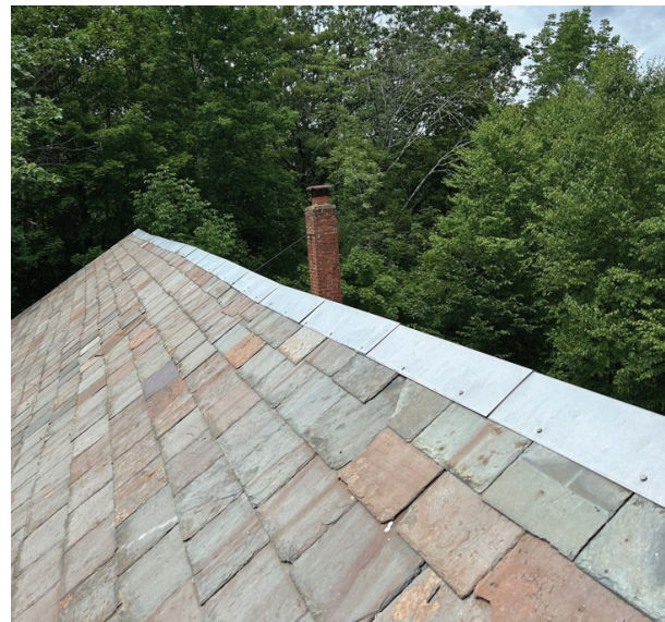
Image A-02: Photo 2 slate detail shows weathered and missing slates and copper ridge cap
