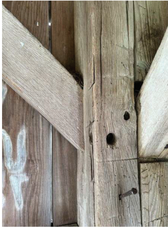
Photo 25 Missing peg from connection
